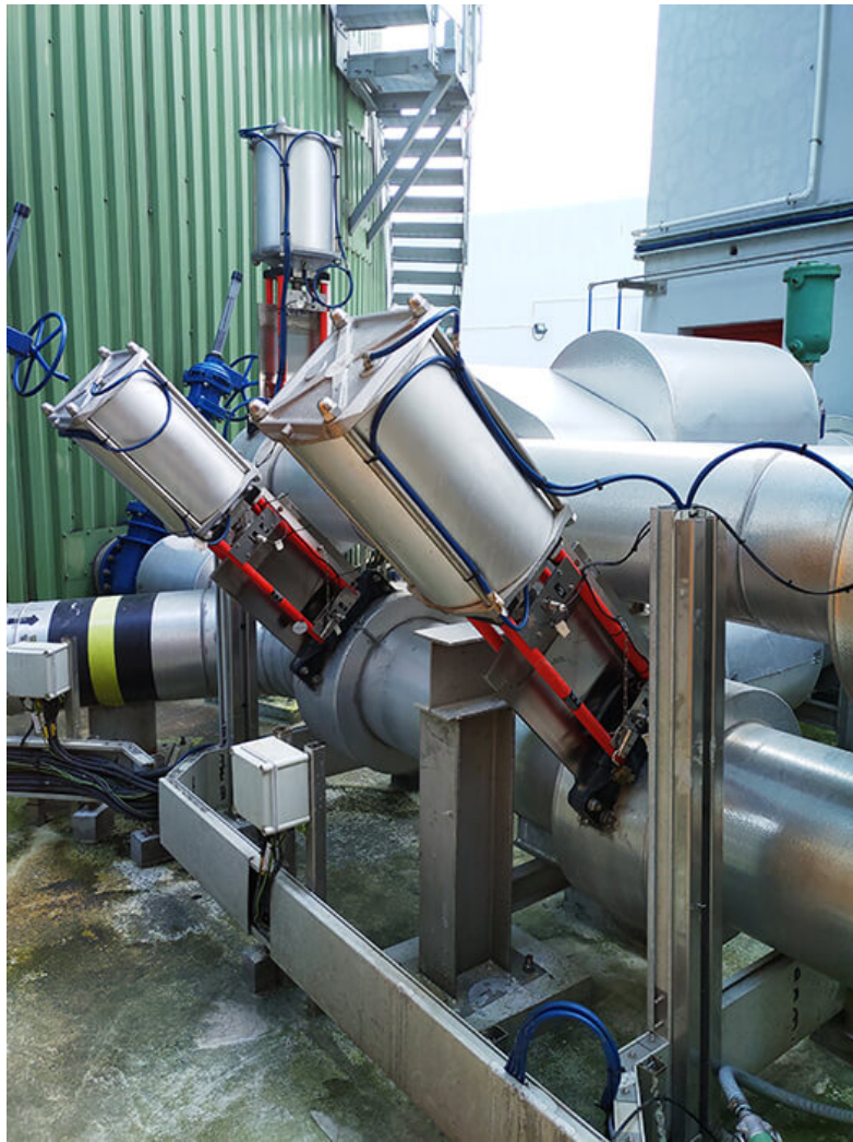
Wey MGC DN 300 in an organic resources recovery centre in Hongkong.
